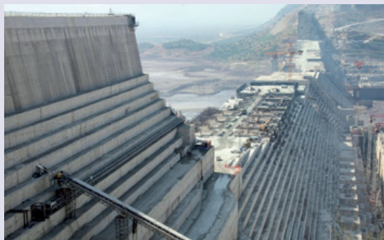
The Grand Ethiopian Renaissance Dam under construction in Nov 2017 (Alamy licenced use for BHS newsletter)
