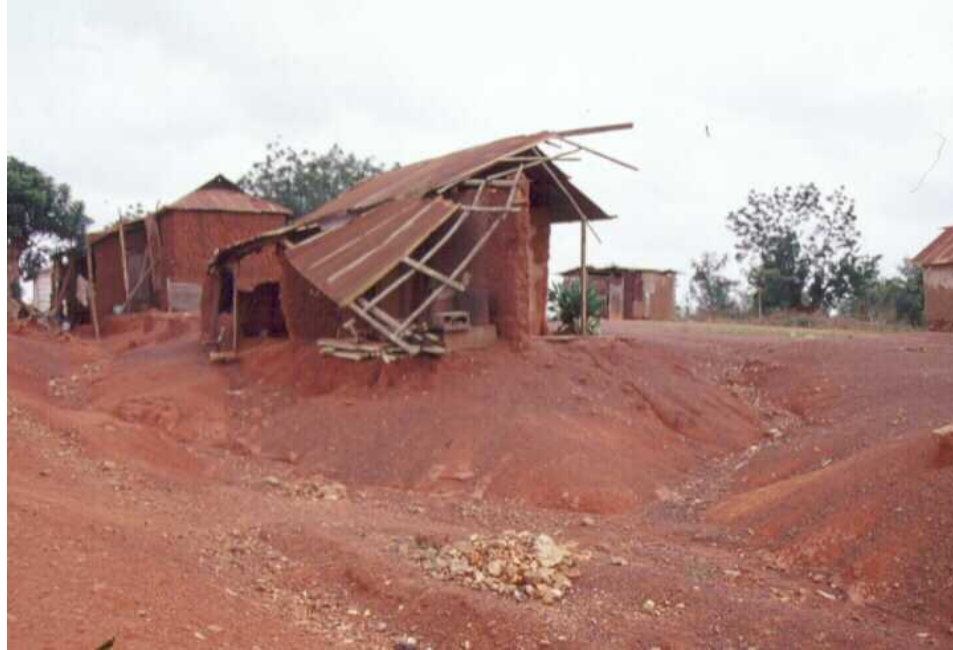
Figure 12. Extensive gulying on the Eastern section of Abora village
