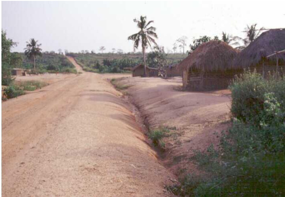
Figure 5. Road-side drain over-deepening due to surficial erosion, Adabra village looking South.
