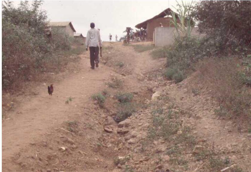
Figure 25. Gully at the start of path 1, Awurabo village. Some gully control may have been undertaken with rock placement.
