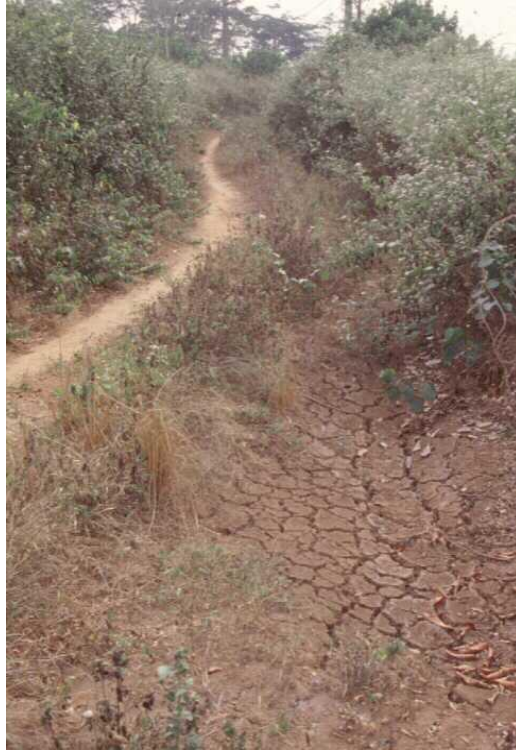
Figure 26. A section of Path 1 (Awurabo village) widened by a tracked vehicle, showing signs of swelling clays (i.e., instability) and gullying
