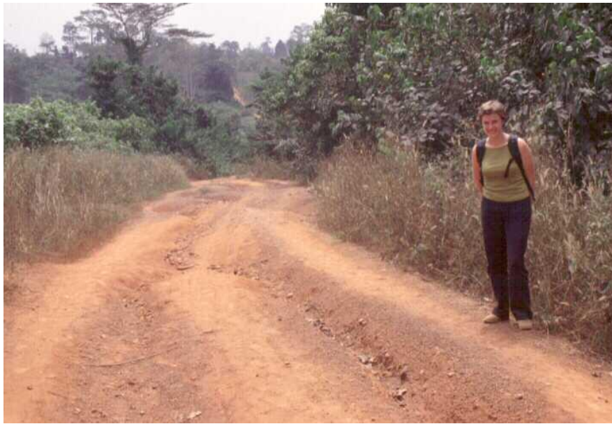
Figure 24. A heavily gullied section of feeder road near to Awurabo village
